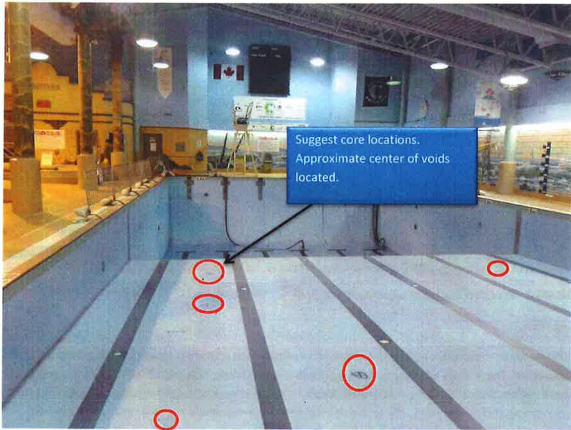
Figure 6: Areas of potential void pockets displayed in the shallow end of the lap pool.
