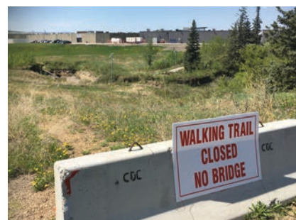
Location of washed out bridge.
