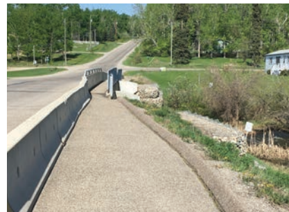
Existing narrow pedestrian crossing at Fish Creek Bridge.
