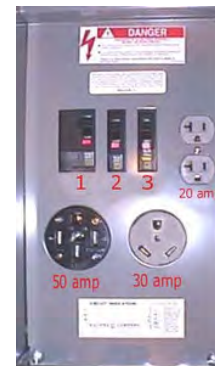
Example of a 20-30-50 electrical hook-up pedestal
