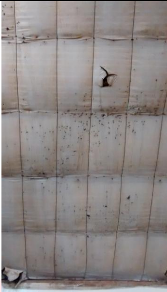
Mold on Ceiling Membrane
