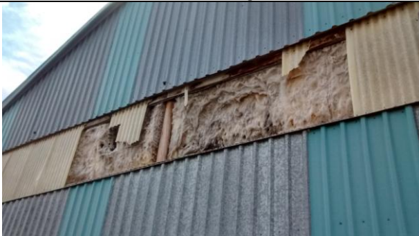
S Wall Broken Fiberglass Sheet (1)
