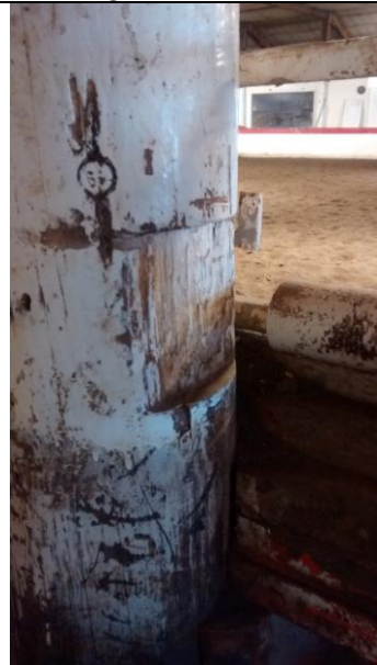
Damage to Column A8
