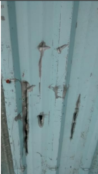
E Wall Cladding Damage
