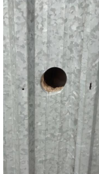
E Wall Unsealed Pipe Penetration
