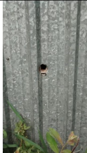
E Wall Unsealed Pipe Penetration (2)
