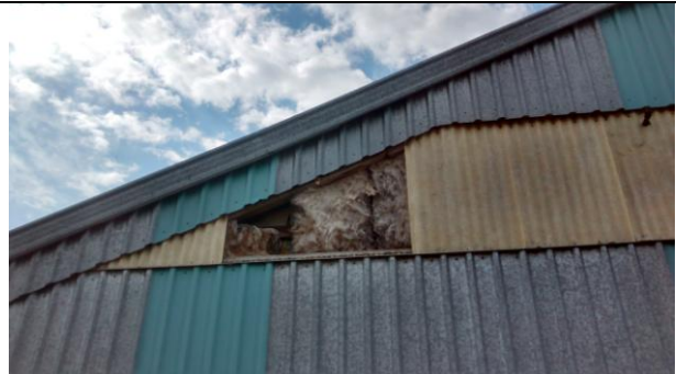
S Wall Broken Fiberglass Sheet (2)
