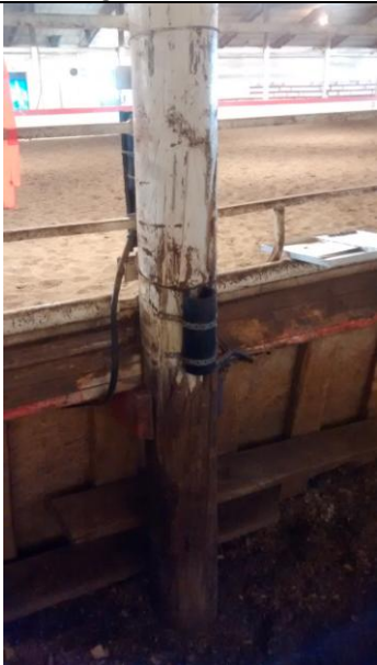
Damage to Column A13
