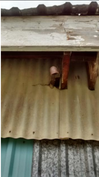
E Wall Pipe and Unsealed Penetration
