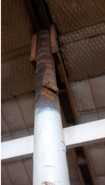
Damage to Column A16
