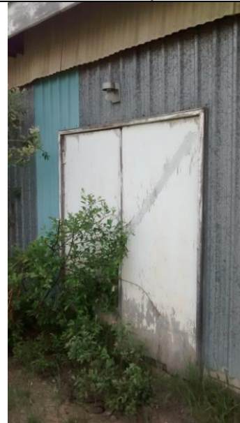
E Wall Blocked Exit
