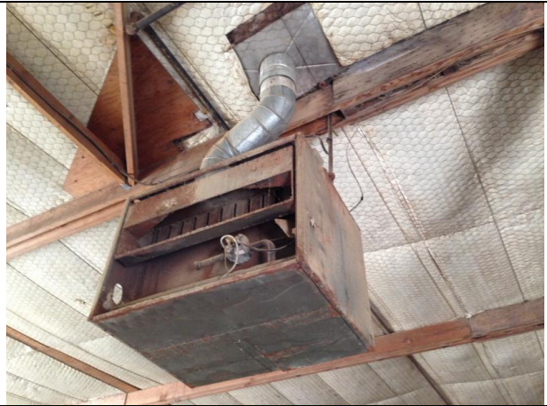
Unused Heating Unit
