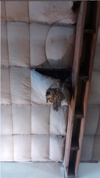
Damaged Ceiling Membrane
