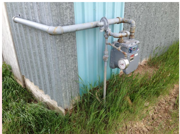
Gas Line – NE Corner of Arena
