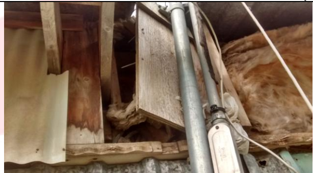
Roof Penetration @ Electrical Connection (3)
