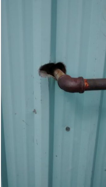
E Wall Unsealed Pipe Penetration (1)
