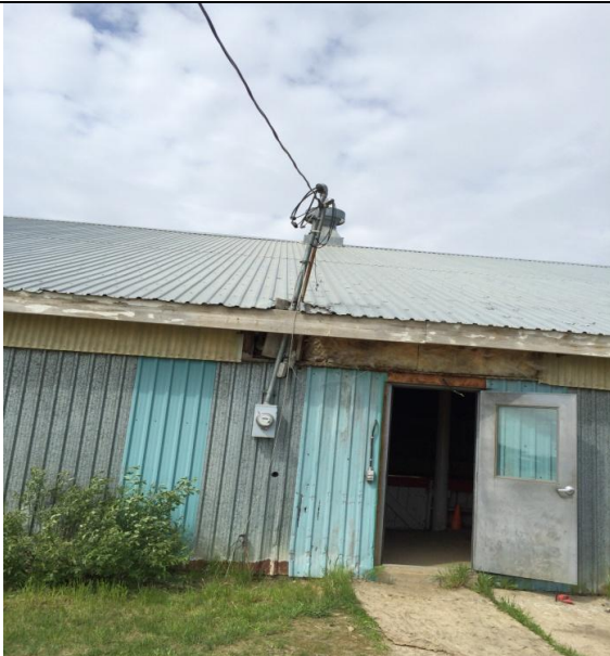
Poorly Supported Electrical Conductor
