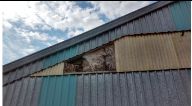
S Wall Broken Fiberglass Sheet (2)
