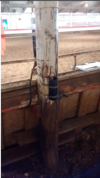
Damage to Column A13
