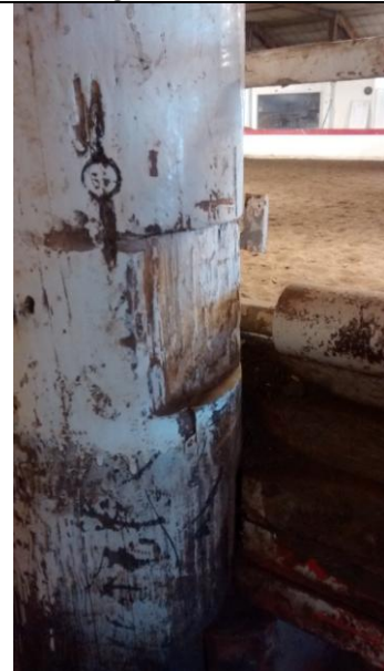
Damage to Column A8
