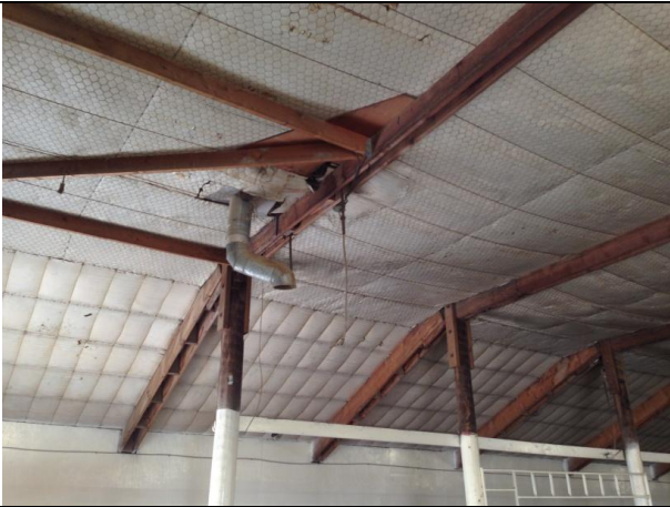
Unused Piping in Ceiling
