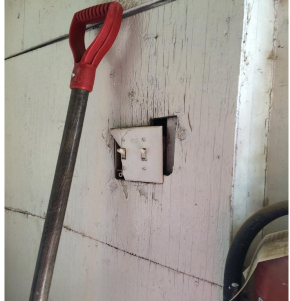
Broken Switch Covers
