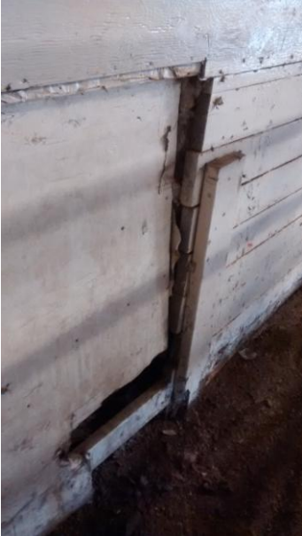
Broken Wall Sheathing (1)
