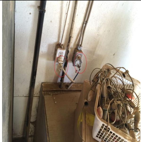
Water Pump Cable
