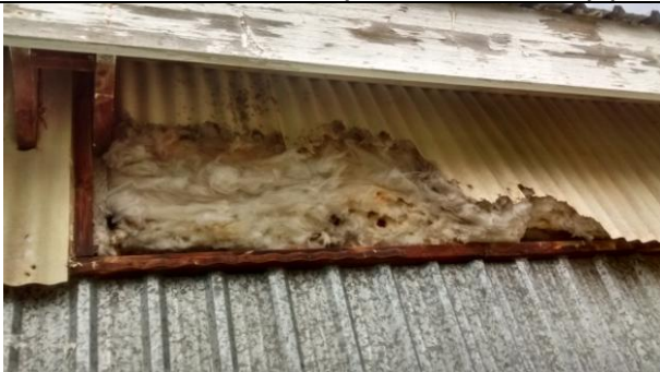
E Wall Broken Fiberglass Sheet
