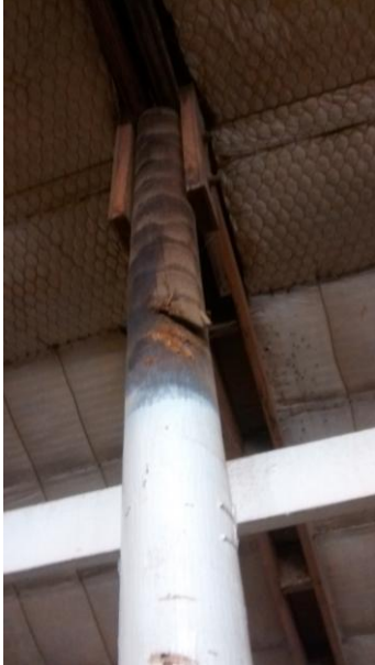
Damage to Column A16
