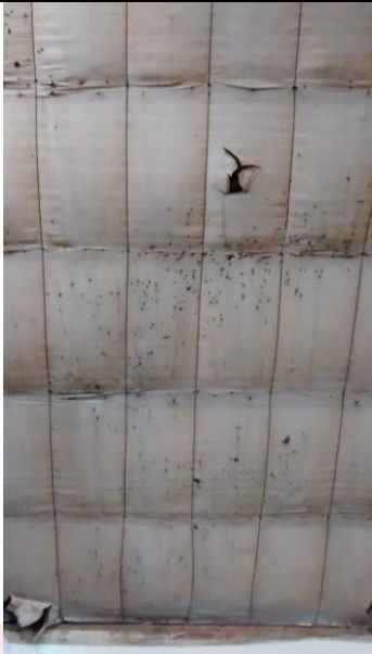
Mold on Ceiling Membrane
