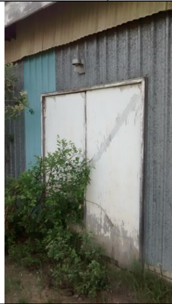
E Wall Blocked Exit
