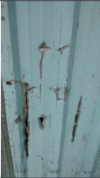
E Wall Cladding Damage
