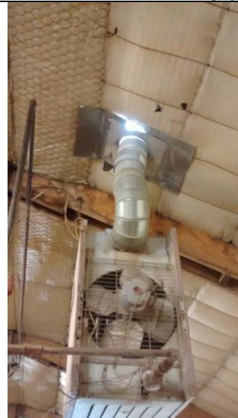
Daylight Through Heating Unit Exhaust
