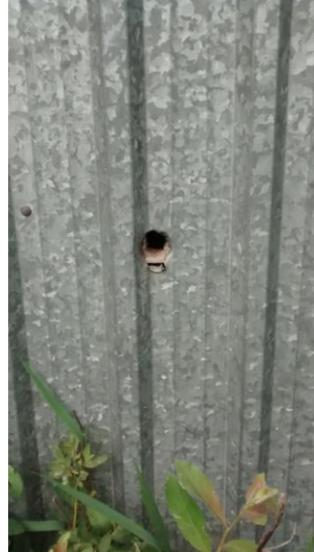
E Wall Unsealed Pipe Penetration (2)
