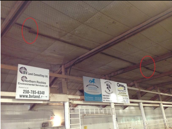
Disconnected Gas Lines
