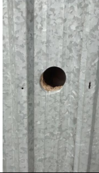
E Wall Unsealed Pipe Penetration
