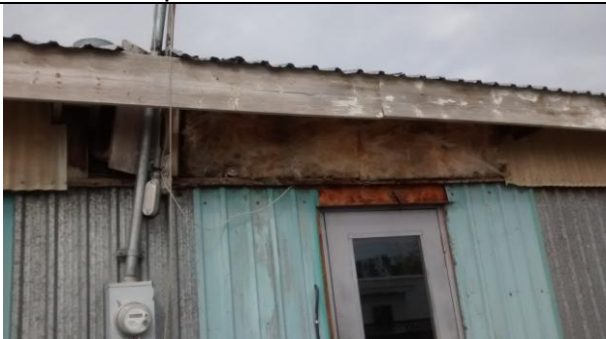
Roof Penetration @ Electrical Connection (2)
