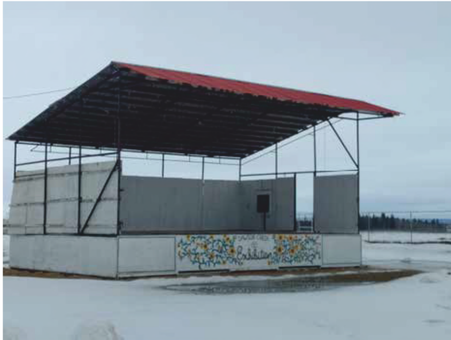
Stage Overall, Showing Minimal Lateral Force Resolution, Failing Backdrops
