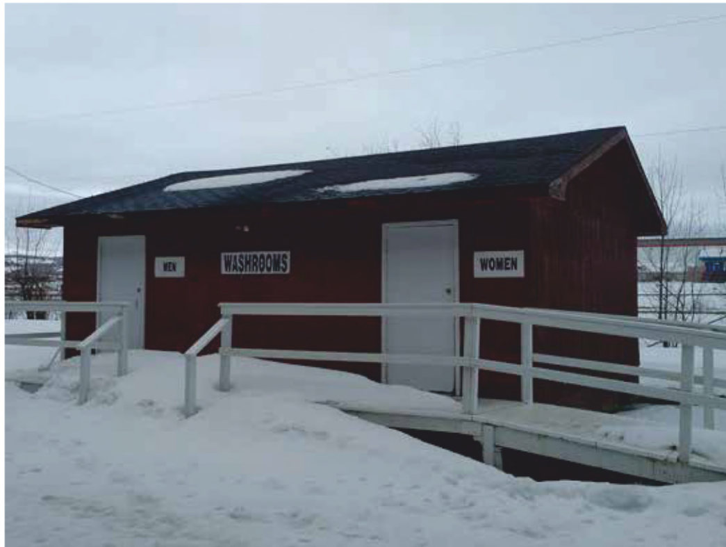
Washroom Building Overall, noting Rotting Eave at Left
