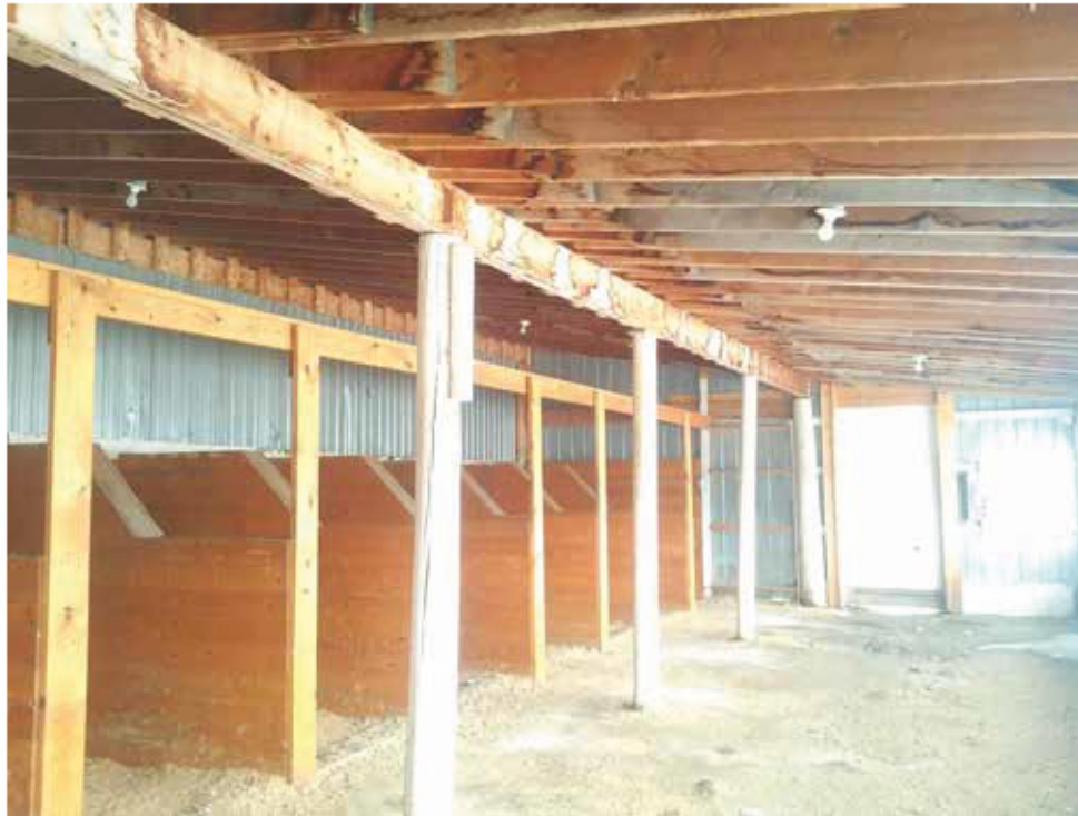
North Lean To Addition, Similar Connection Issues to South
