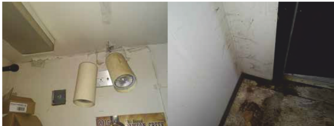
Roof Leaks and Deteriorating Floor Areas Noted
