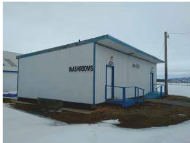
Structure #34, Washroom. Note Settlement of Left Ramp
