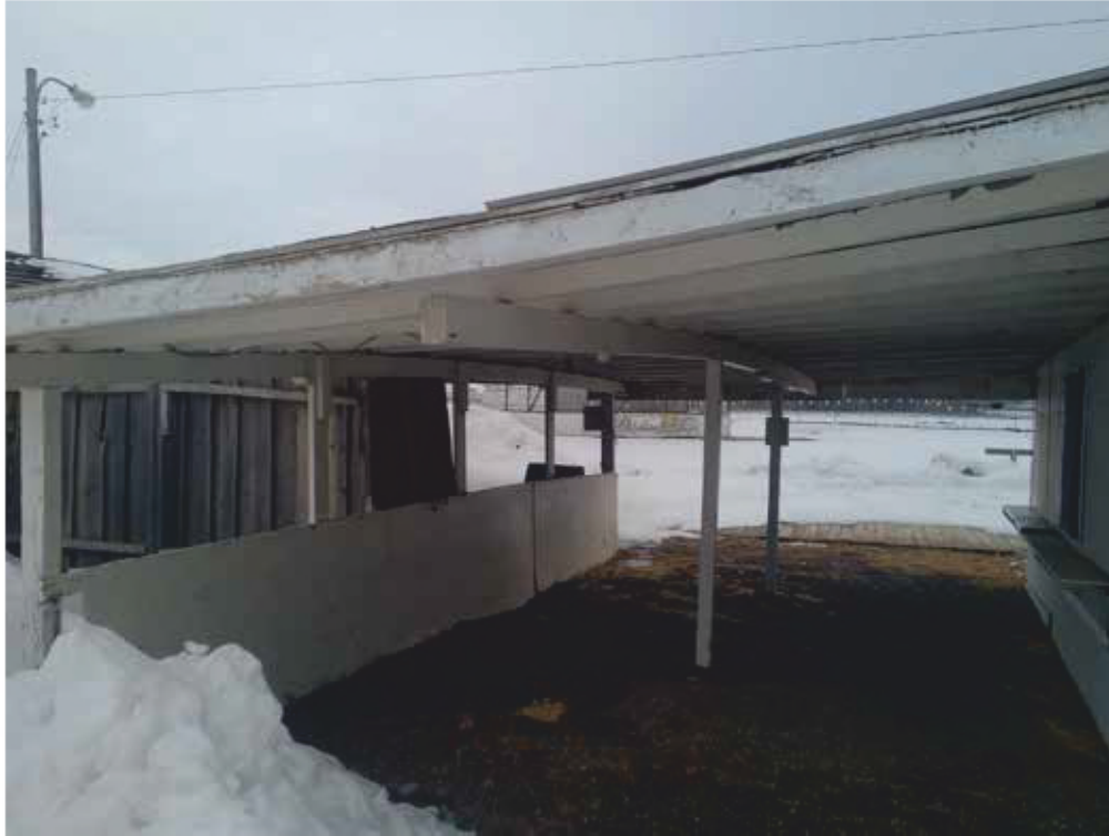
Missing Structural Supports, Highly deformed Structure
