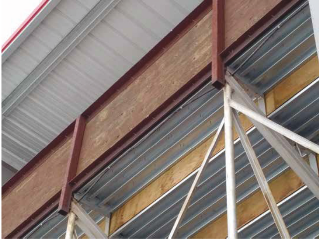
Corroding Safety Barrier Supports and Welds
