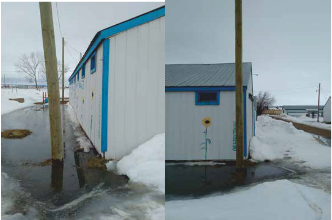
Stable 7.1 – Showing Kicked out South Wall Left and Bulging Gable East End
