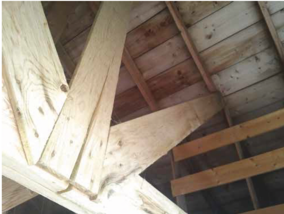
Rafters Breaking At Mid Span Throughout
