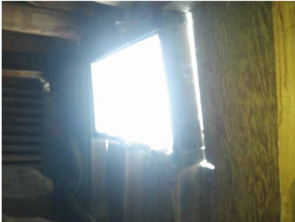
Completely Buckled and Broken Load Bearing Wall
