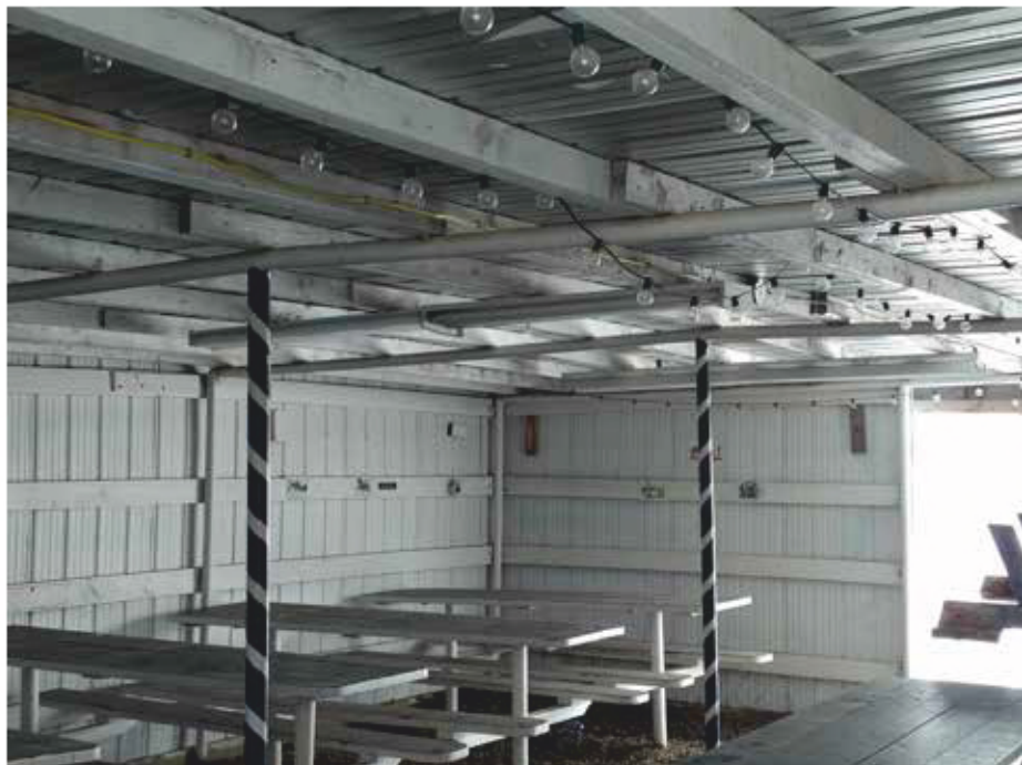
Bent, Distorted, and Poorly Connected Roof Over Seating Area
