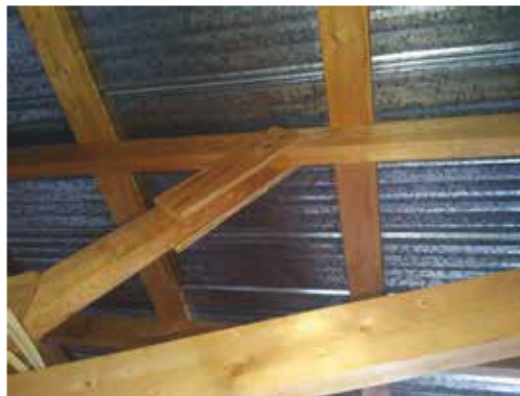
Web Member not correctly Mitred to Chord, Insufficient Nailing
