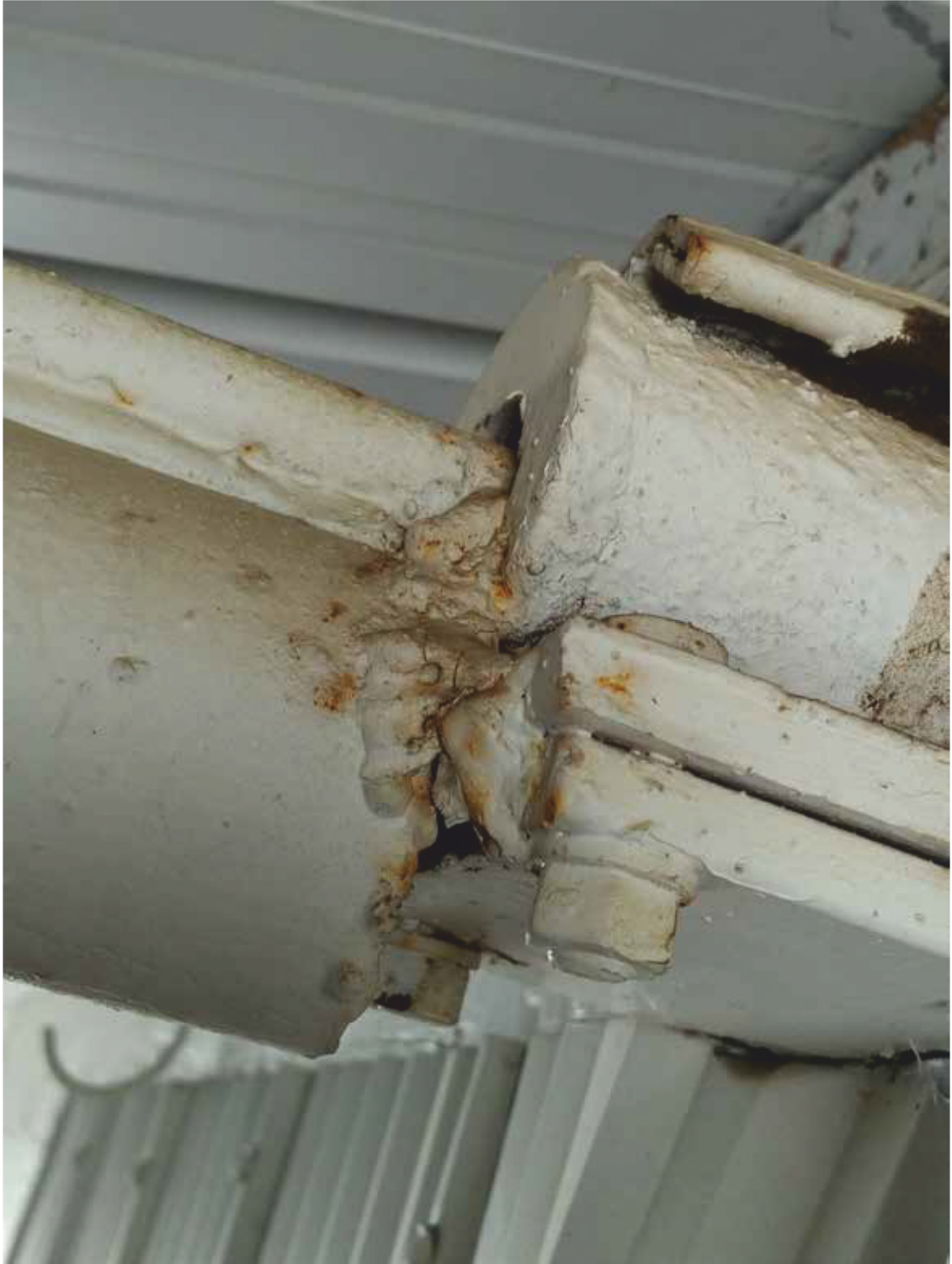
Broken / Cracked Welds Supporting Roof
