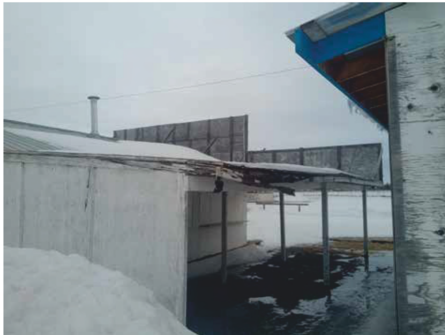
Roof Deterioration Building 'E'
