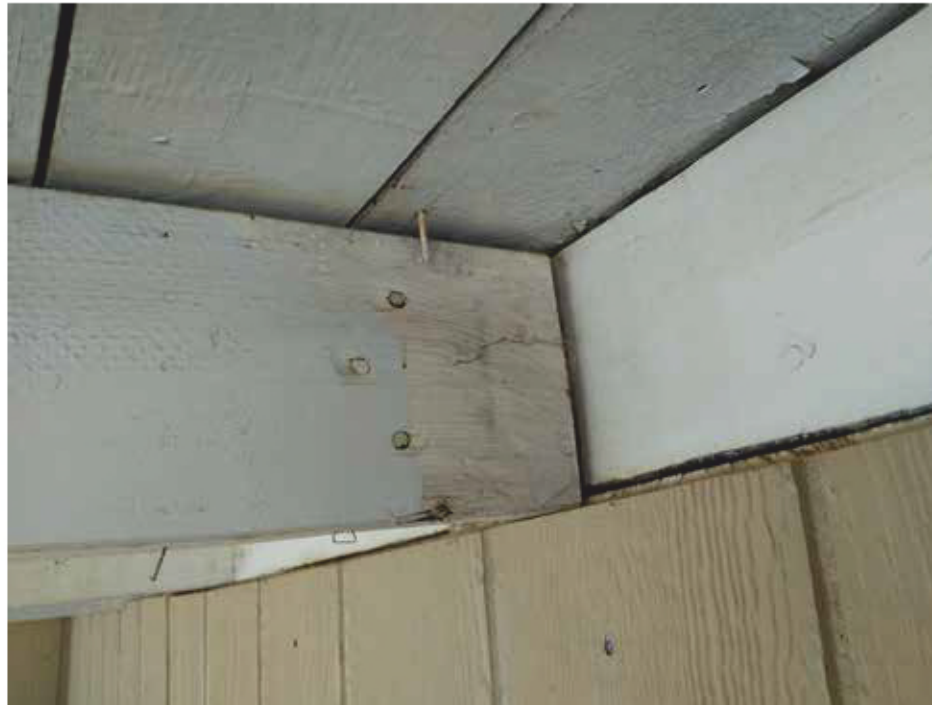
Joist Seat Bearing does not meet Minimum Criteria
