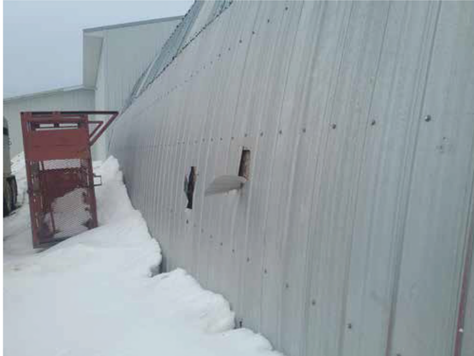
Roof Holes and Snow (Meltwater) Accumulation against Building
