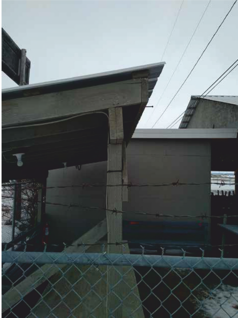
Beam Rolling due to Poor Framing Technique
