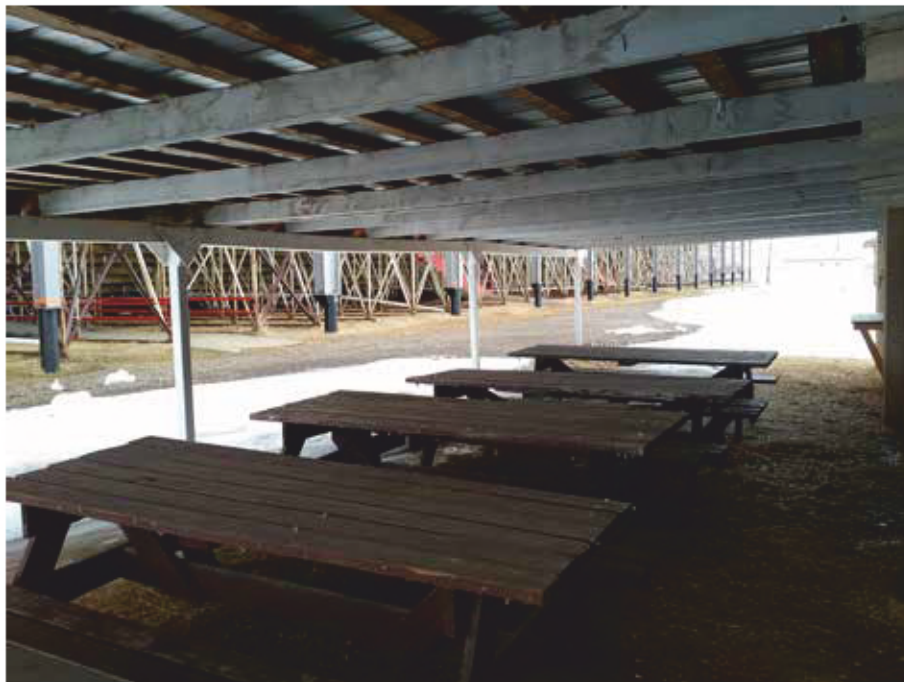
Covered Seating Area Showing Deflected Beams and Joists
