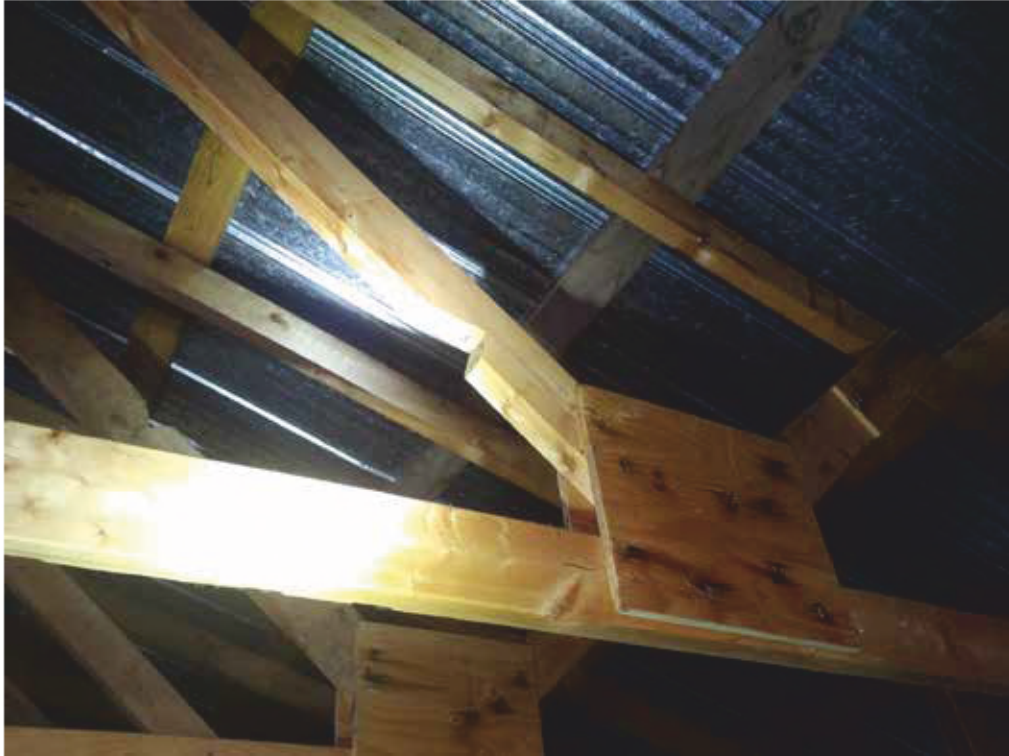
Notched Web Member, Insufficient Plate Nailing
