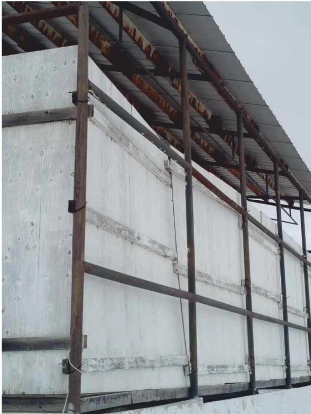
Broken Zip Ties Causing Backdrop Collapse
