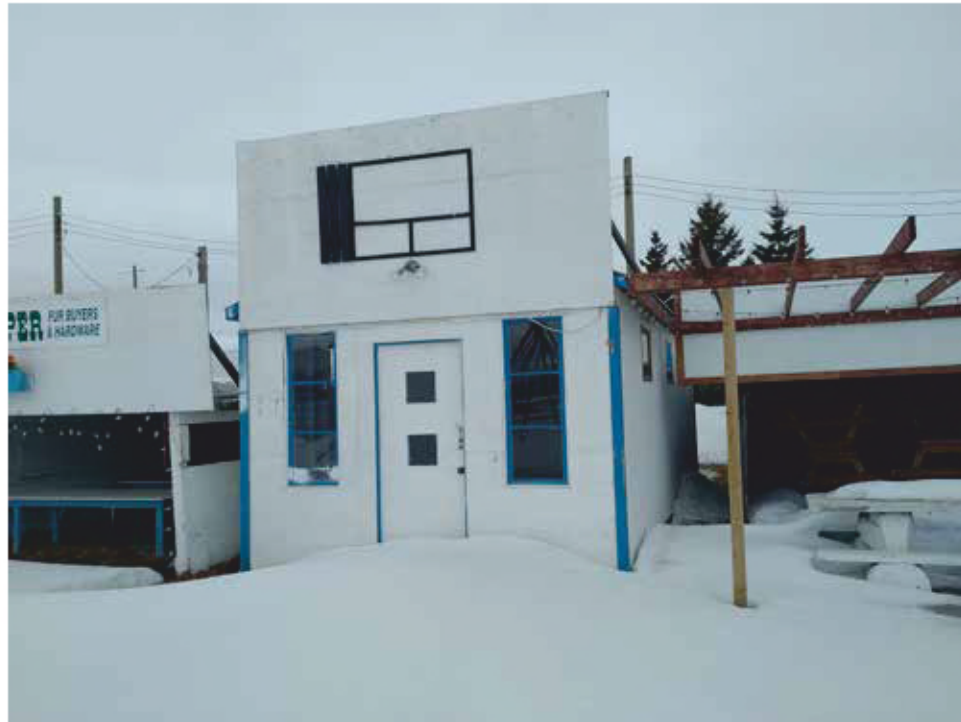
Building 'B' With Poorly Attached False Front
