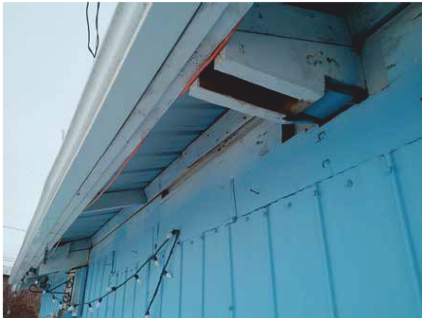
Steel Post / Rafter Connections, not Constructed to Part Nine Standards
