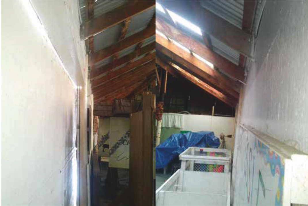
North (Left) and South (Right) Walls Deflecting Outward at Top
