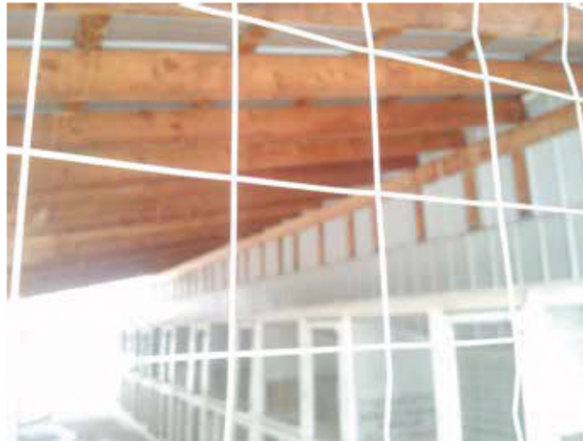
Lean To Structural Connection Made Over Cladding
