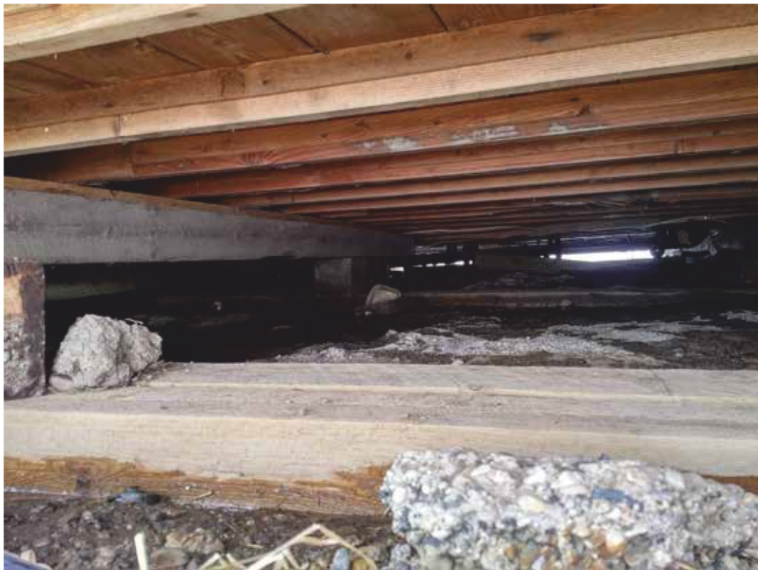
Undersized Floor Framing and Support Timbers Below Structure
