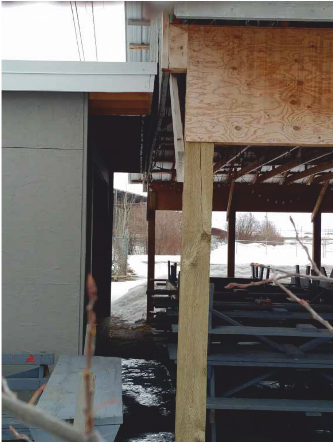
Detail of Construction Showing Buckling of End Gable
