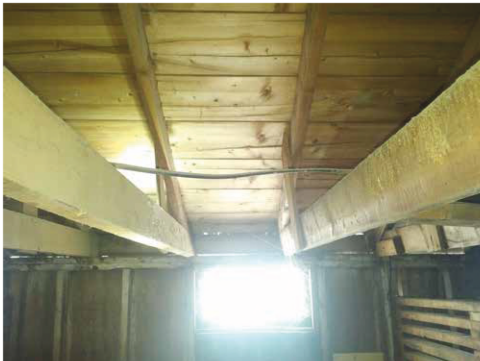
Roof Joists and Ties Rolling over in Near Collapse Condition
