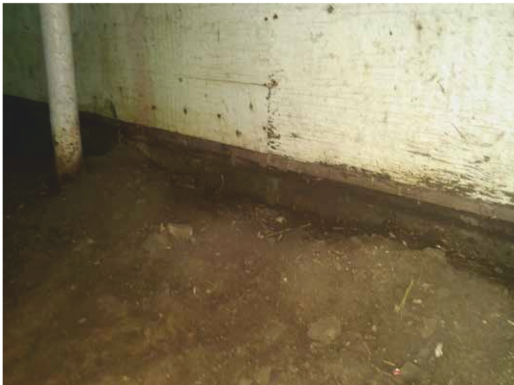
Decay of Wood Members due to Earth Burial
