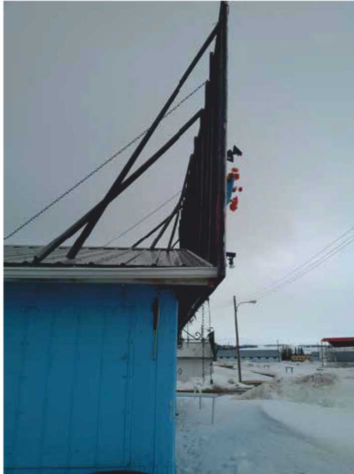
Framing of False Front of Building Failing, Chains Drawn Tight
