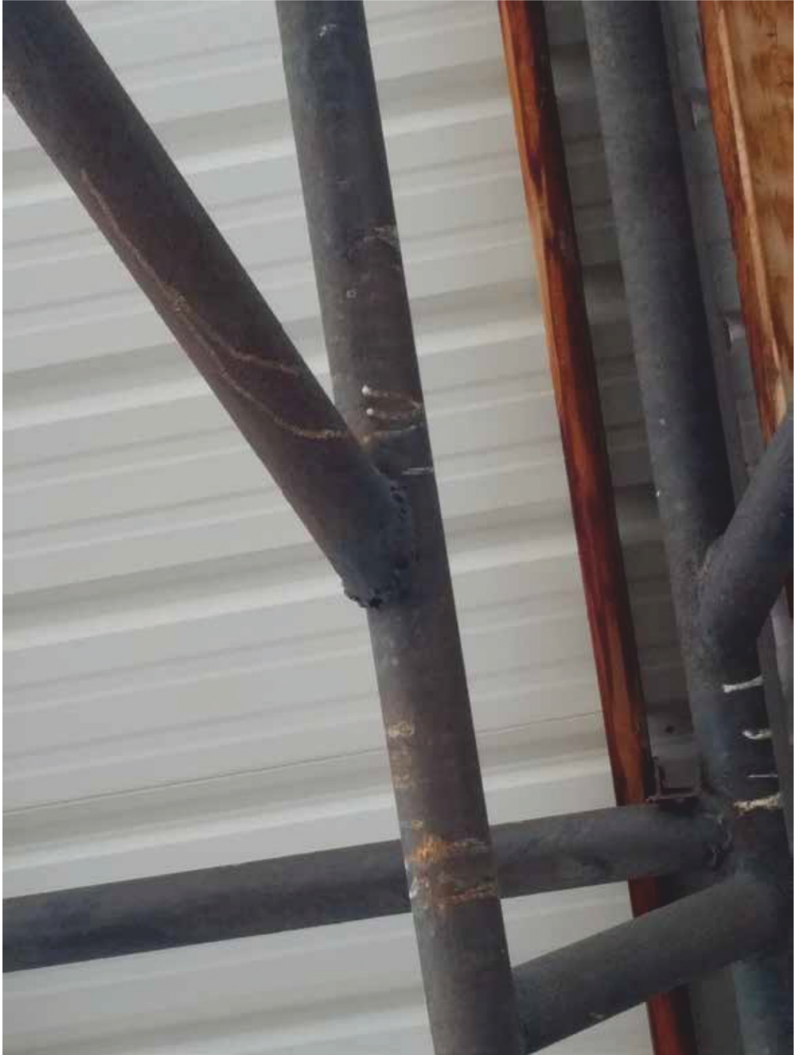
Misalignment and Poor Quality Welds
