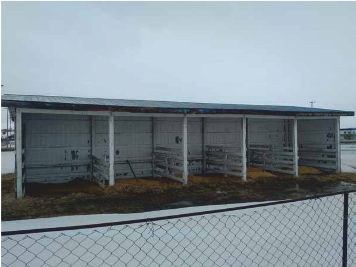
Structure #11, Noting Uneven Settlement Of Posts/Columns
