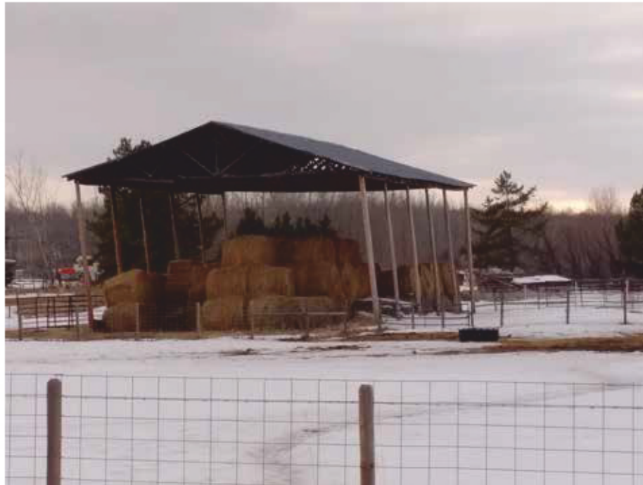
Pole Building Nearing end of Service Life
