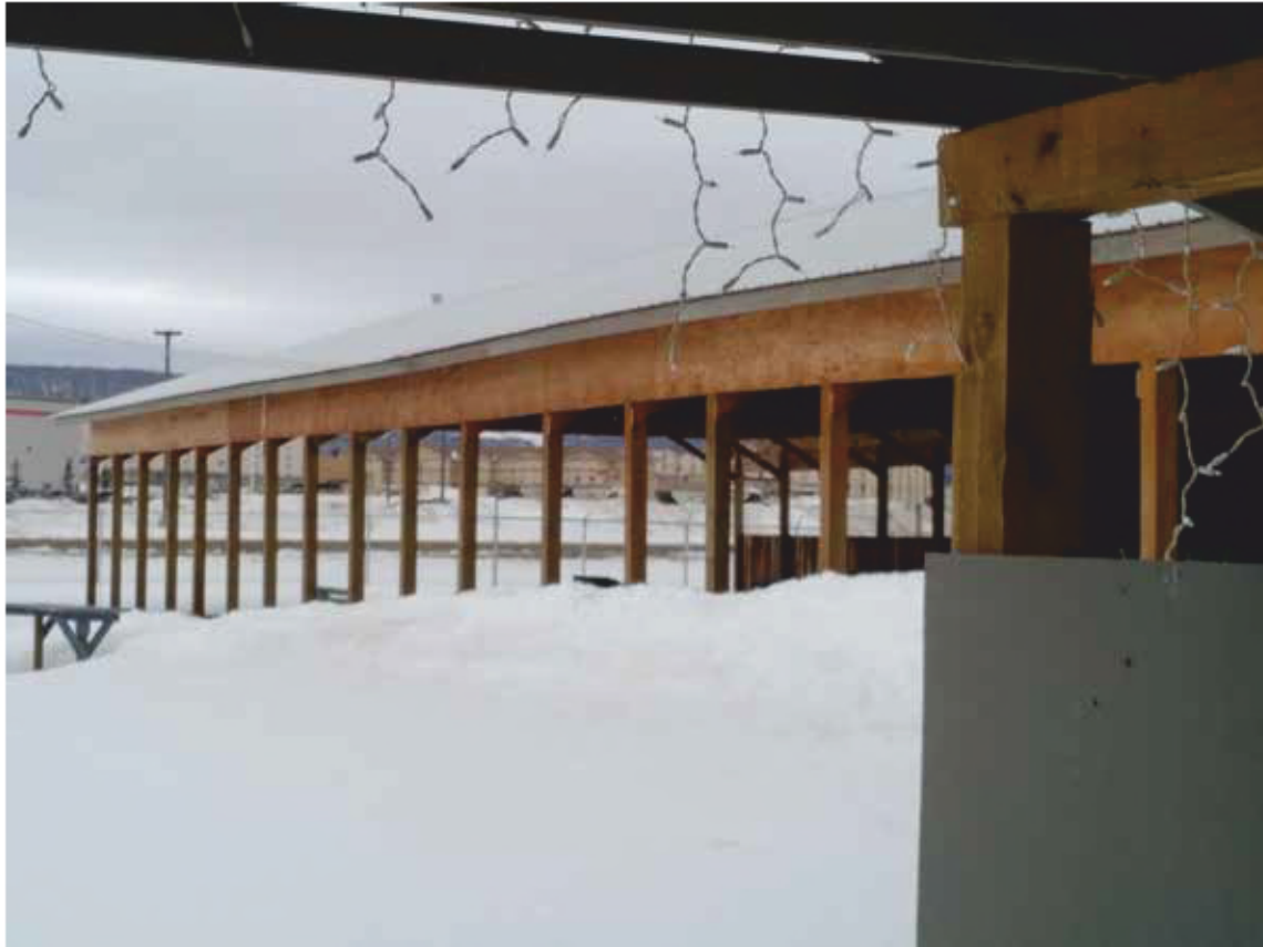
Settlement of Structure Illustrated @ Centre
