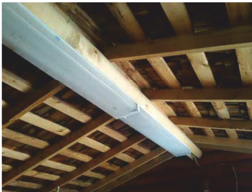
Interior Building 'F', Roof Missing Collar Ties
