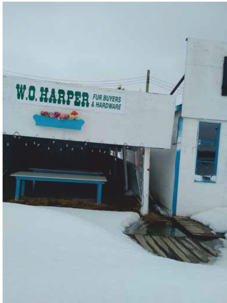
Building 'A' Seating Area Near Collapse
