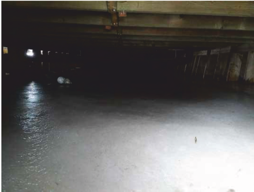
Flooded and Severely Iced Crawlspace Below Washrooms
