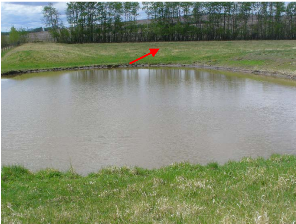
Photo 4 – Gap in low-level (left) dyke at dugout just east of #215 Road allows water to cut across hay field and re-enter Rolla Creek downstream
