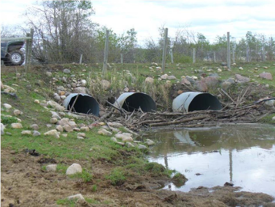
Photo 1 – Rolla Creek Culvert Entrance at Farmyard Crossing – approx. 50% of flow capacity is being sacrificed.
