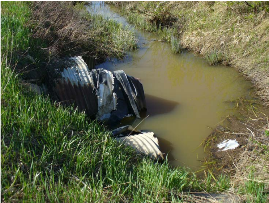
Photo 2 – Rolla Creek – Culvert Entrance at #215 Rd. crossing and roadside channel that makes two 90 deg. Bends, as presently aligned.
