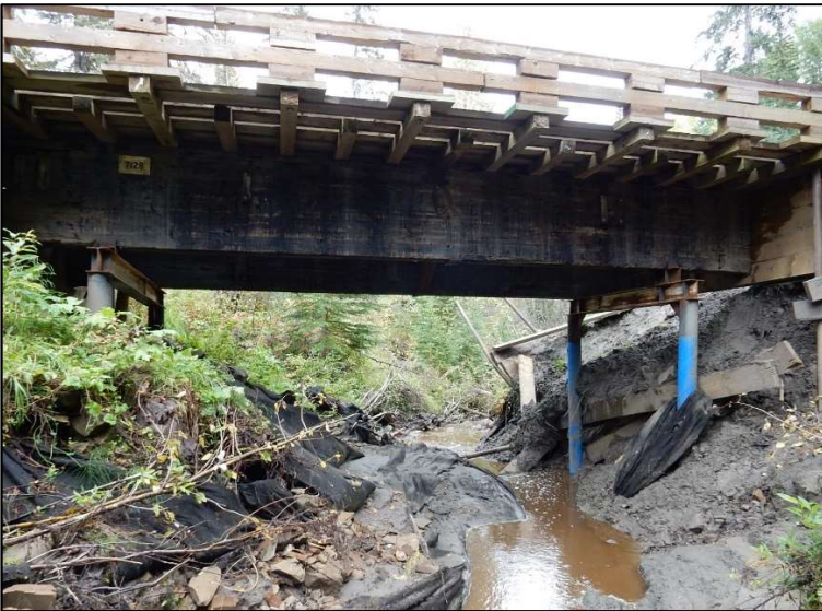
US elevation. RB piles exposed.
