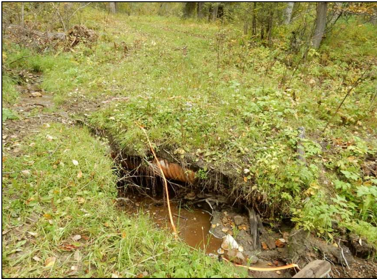
RB approach. Culvert washed out.
