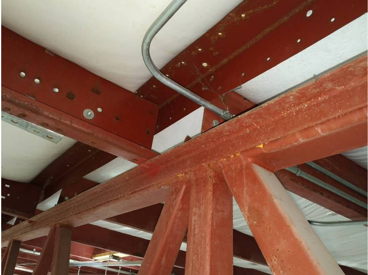
Roof Diaphragm Connection Improvement Required Between Phases
