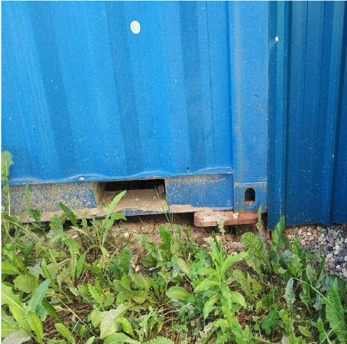
Grade is Sloped Towards Building, Flooding Draintile
