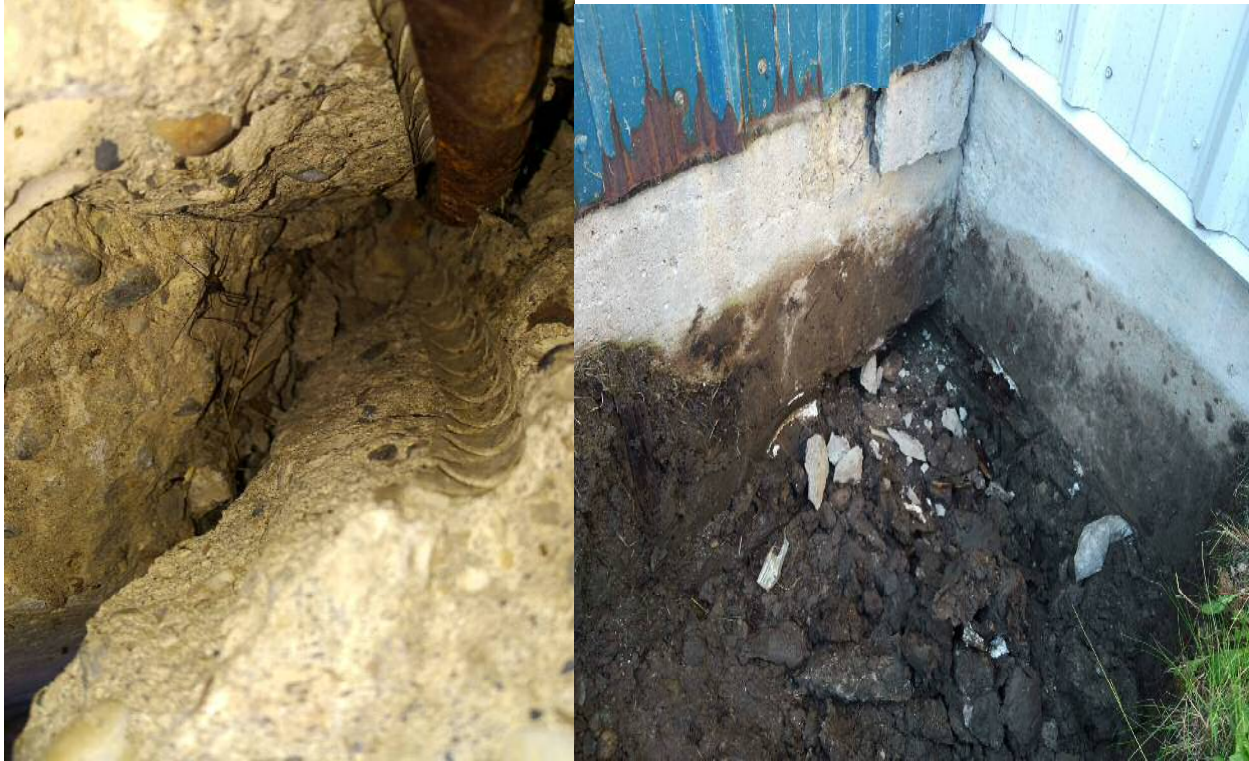
Excavation at Grids 11 and A, Showing Spalled Concrete, and Previous Repair
