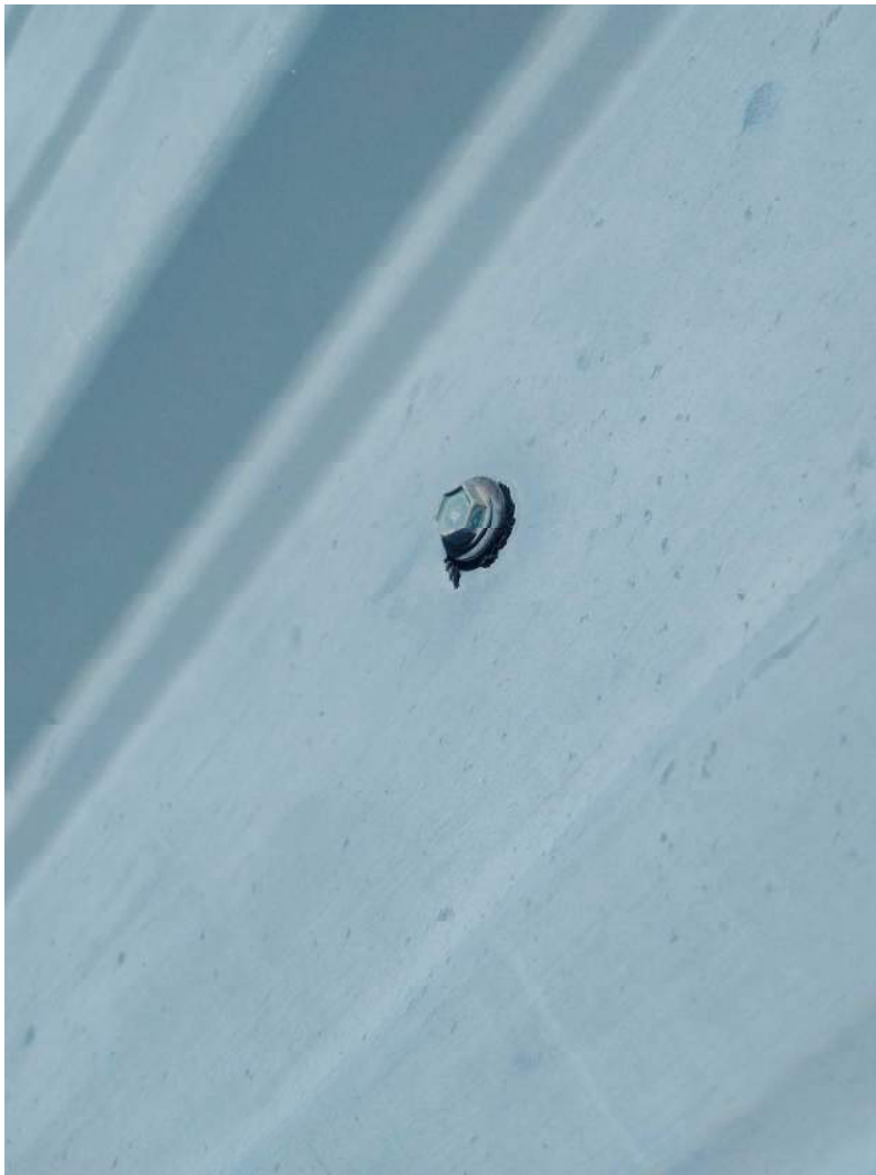
Typical Fastener Washer Degradation Throughout
