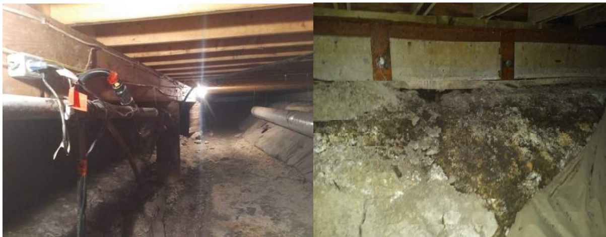
Crawlspace General and Perimeter Grade Sloughing
