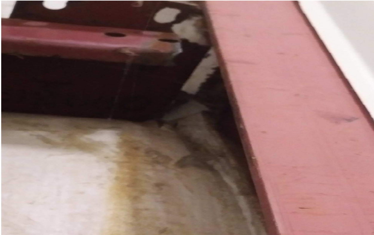
No Apparent Connection Between the 1975 and 1989 Buildings
