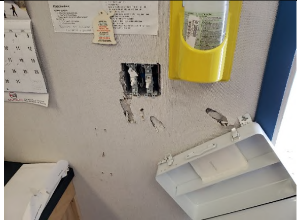
Photo 7: Damage to equipment at Cecil Lake Transfer Station.
