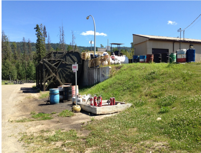
View of the Transtor Units and Retaining Wall
